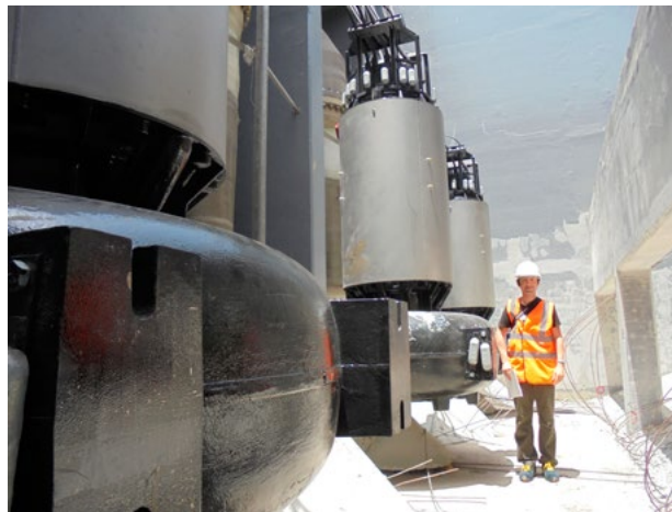
Gabriele Casella at the Al-Khumra pumping station
