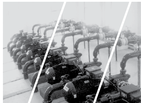
Boosting and Distribution of surface water
