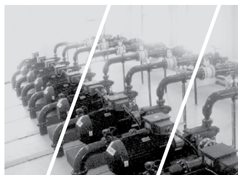
Boosting and Distribution of surface water
