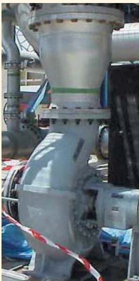
Below: Cooling water pump for primary turbine at a power plant in the Middle East.
