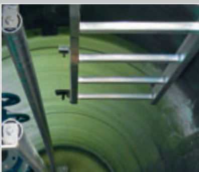
Built-in service ladder.
