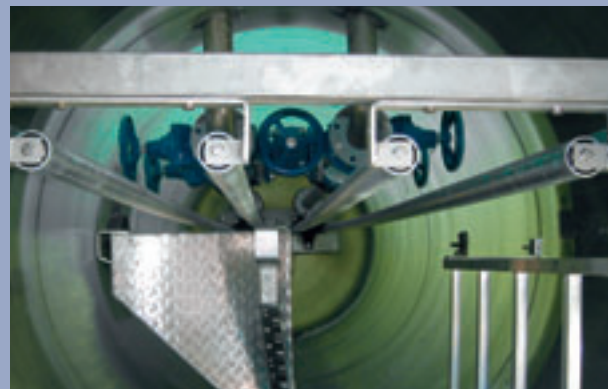
Customised pipe configuration with two separate discharge pressure pipes.
