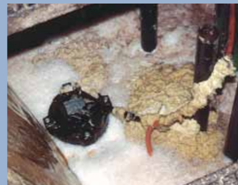
One of two S pumps used at a glass wool manufacturing plant for pumping process water with a high content of abrasive particles.
